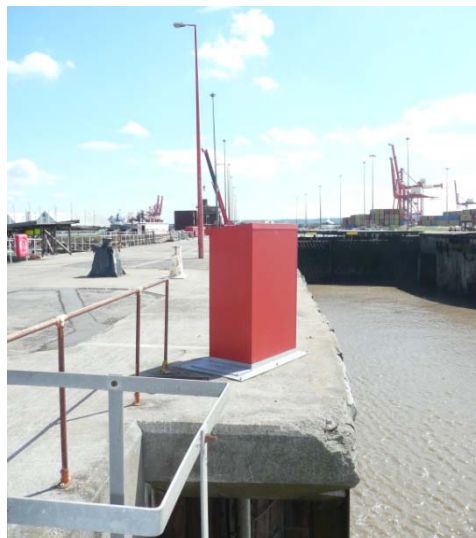
Portbury Tide Gauge Cabinet
